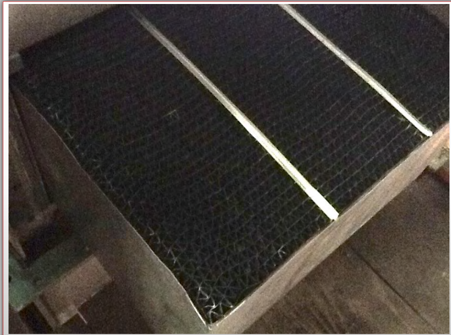
Top View of Module Removed for inspection
